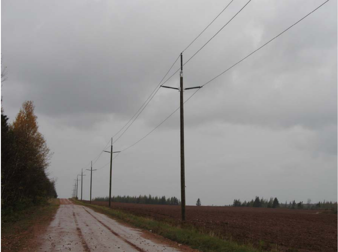
Figure 1. Photograph of transmission line.
