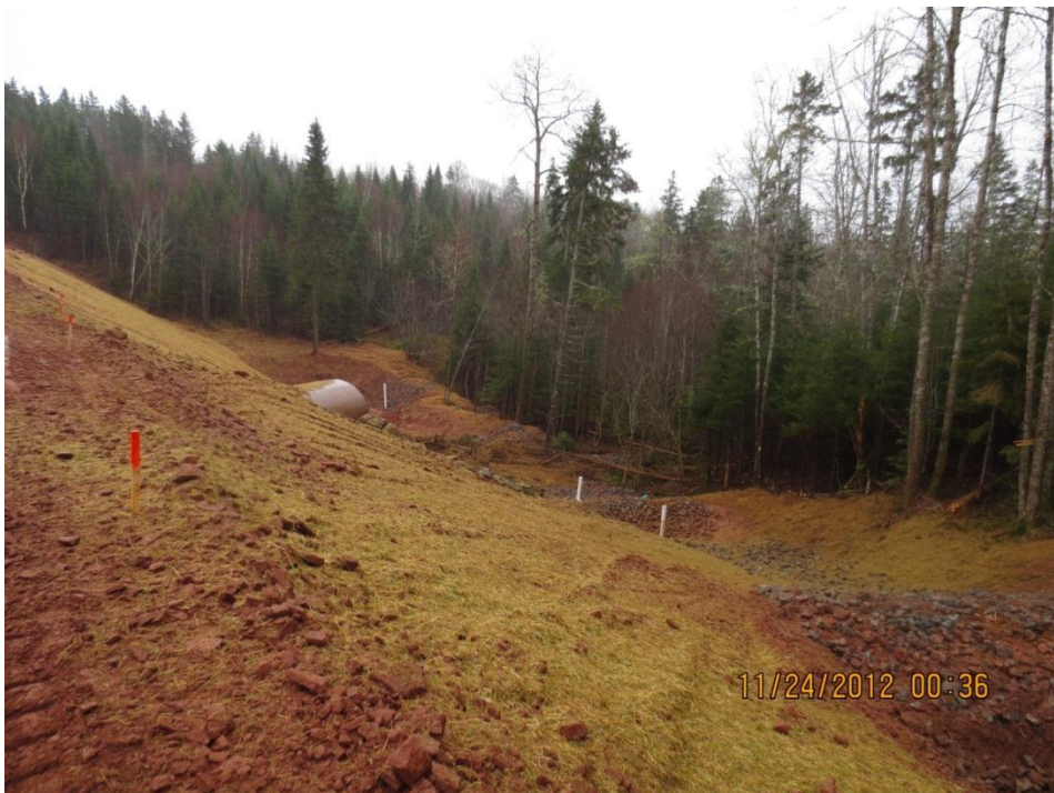
PHOTO 10: Mulched slopes at Encounter Creek (Station 2+450, facing southeast) on November 24, 2012, following installation of concrete pipe.
