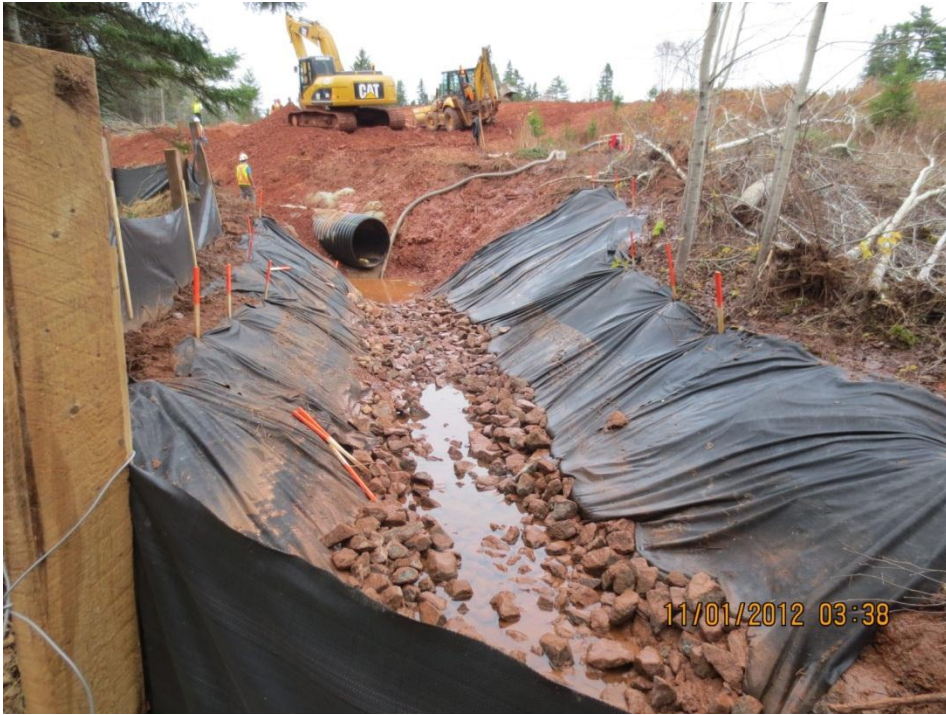
PHOTO 19: Installation of stream diversion channel at Crawford's Stream (Station 1+500, facing north), November 1, 2012.
