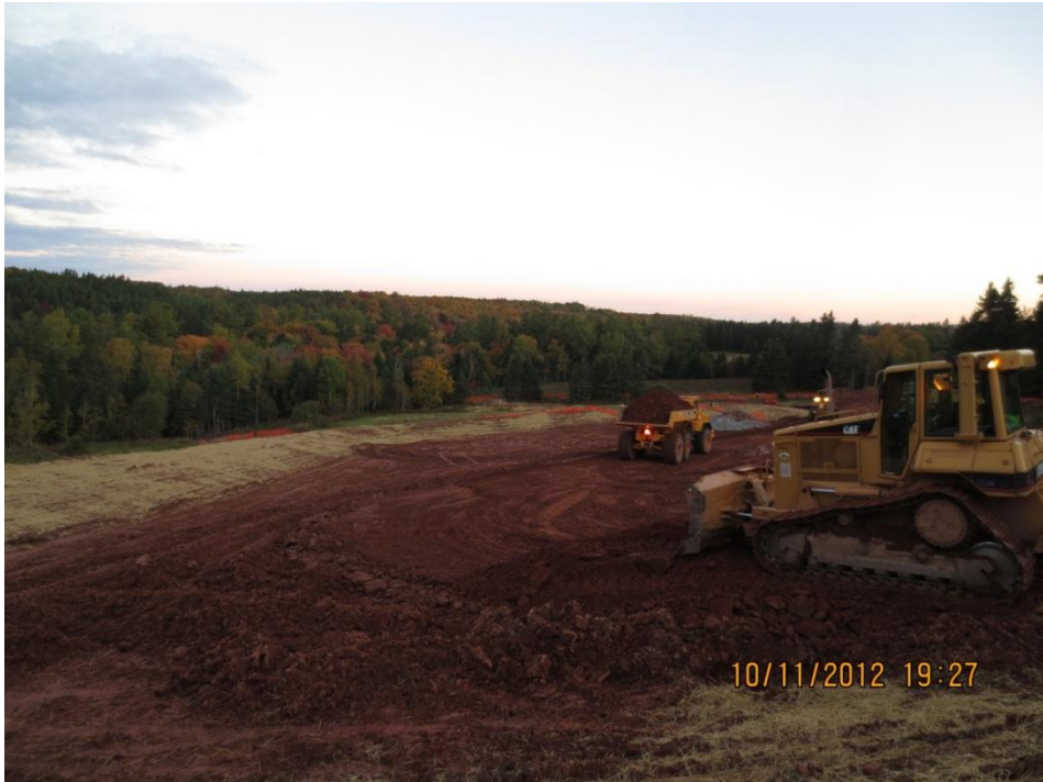
PHOTO 13: On-going construction of staging area at Crawford's Stream (Station 1+600, facing north), October 11, 2012.
