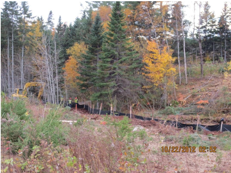
PHOTO 18: Installation of silt fence for stream diversion channel at Crawford's Stream (Station 1+520, facing southwest), October 22, 2012.
