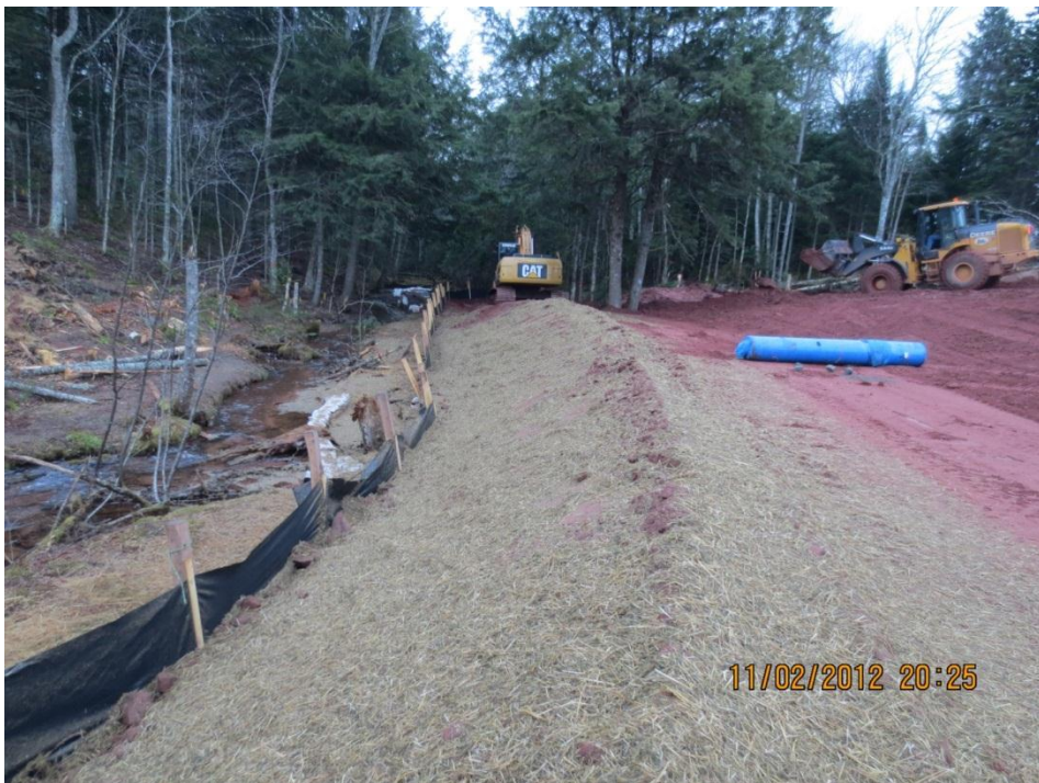
PHOTO 20: Preparation of stream diversion channel at Crawford's Stream (Station 1+500, facing north), November 1, 2012.
