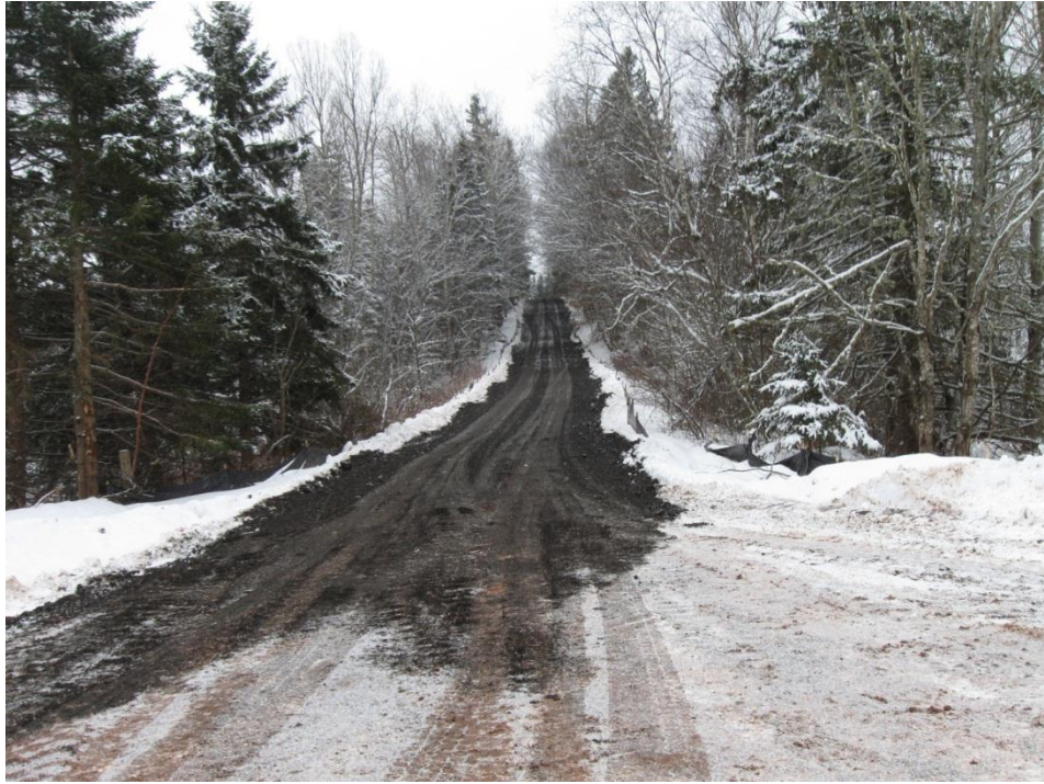
PHOTO 29: Newly placed reclaimed asphalt pavement on Peter's Road (adjacent to Crawford's Brook construction area, Station 1+025, facing south) for winter stabilization, late December 2012.
