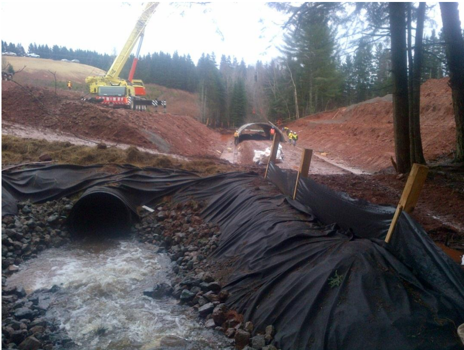
PHOTO 22: Stream diversion channel and on-going construction of concrete arch at Crawford's Stream (Station 1+500, facing south), December 11, 2012.
