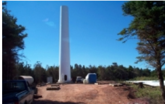
Construction at the new wind farm at North Cape. The facility will supply power to provincial and federal office buildings in PEI.
