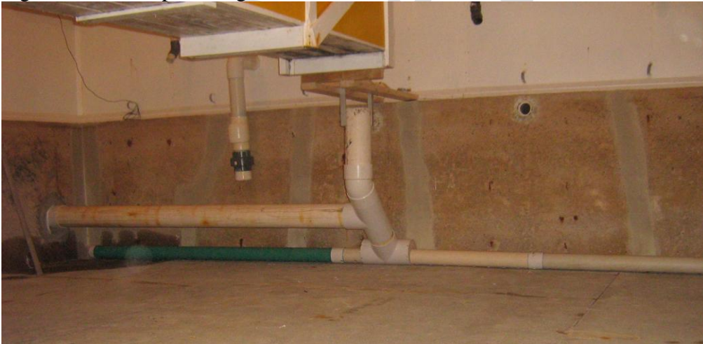
Figure 18: Drain plumbing for Tank 1B
