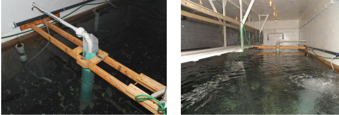
Figure 24 a, b: Pump sleeve piping and placement for foam fractionator feed
