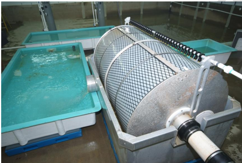
Figure 19: Drum filter for effluent water
